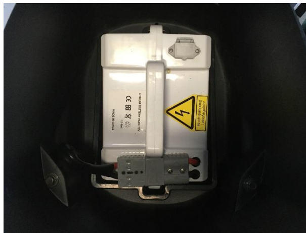
Discharge plug connected
